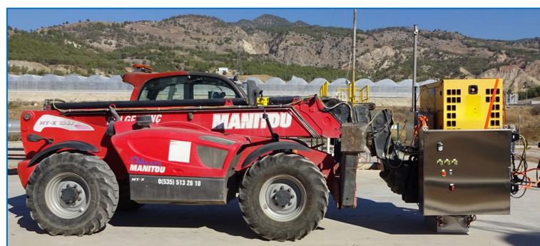
Figure WP4.10: C: Field implementation of 10kN at Kilzildere geothermal plant.
