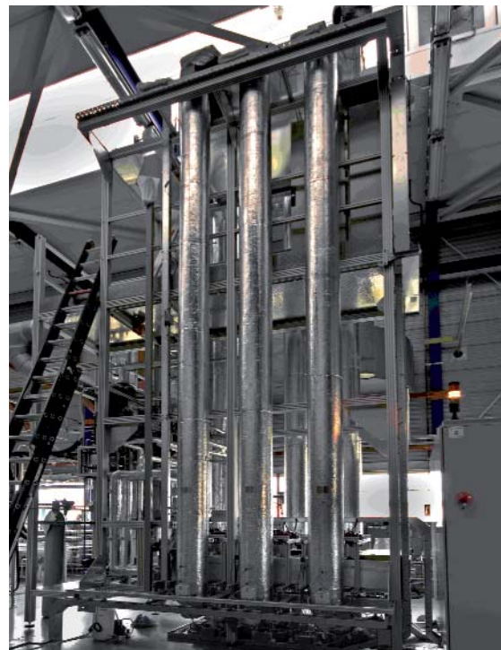
Figure 3.3 SEWGS six-column pilot unit.
