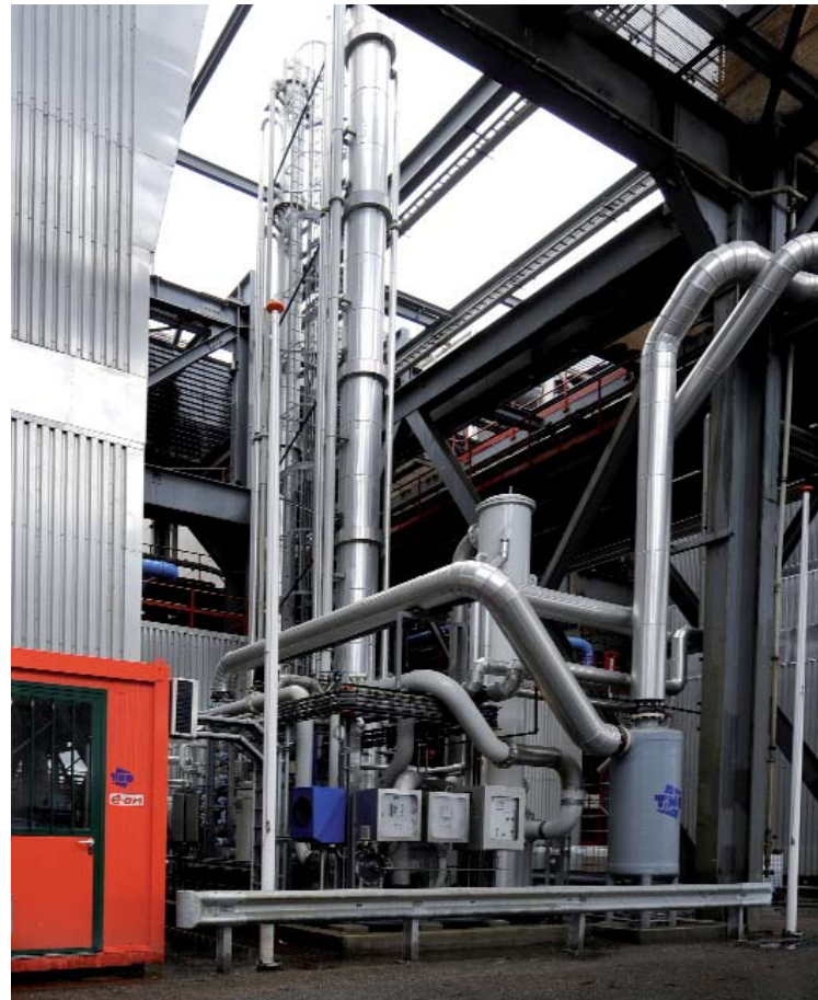
Figure 3.1 CATO CO 2 Catcher at the coal-fired power station of E.ON.
