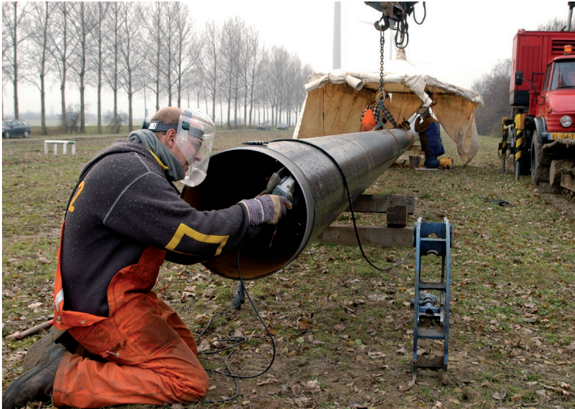
| Work on the CO 2 pipelines of OCAP in the Rotterdam area. Picture: Hans de Lijser.
