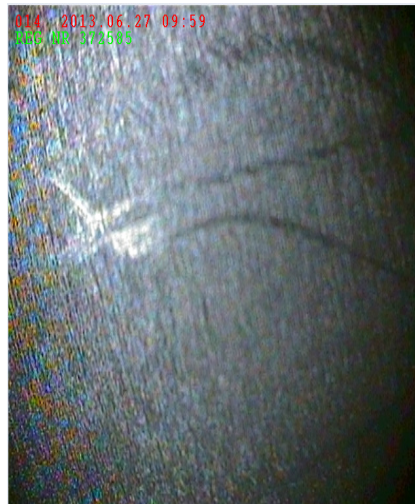
pipe at elevation +4500
