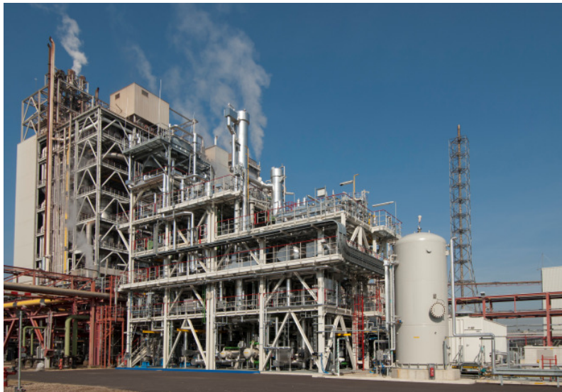
Figure 2-5: CO 2 capture pilot plant. The tall column in the middle of the picture is the CO 2 absorber.
