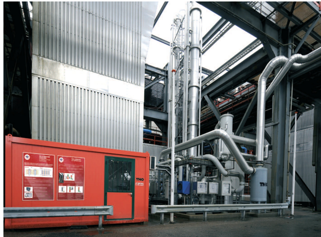
Figure 2-1: The TNO pilot capture plant at the EOn site at the Maasvlakte (Rotterdam, the Netherlands)
