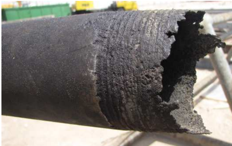
Figure 4.2. A pin and box coupling failure due to H 2 S gas (1000 ppm) + 2% CO 2 .
