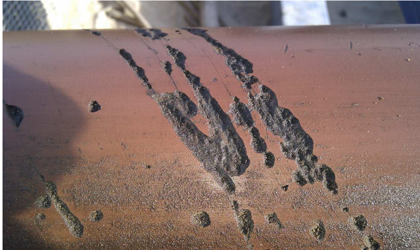
Figure 4.3. A pipe corroded due to H 2 S gas (1000 ppm) + 2 % CO 2 .
