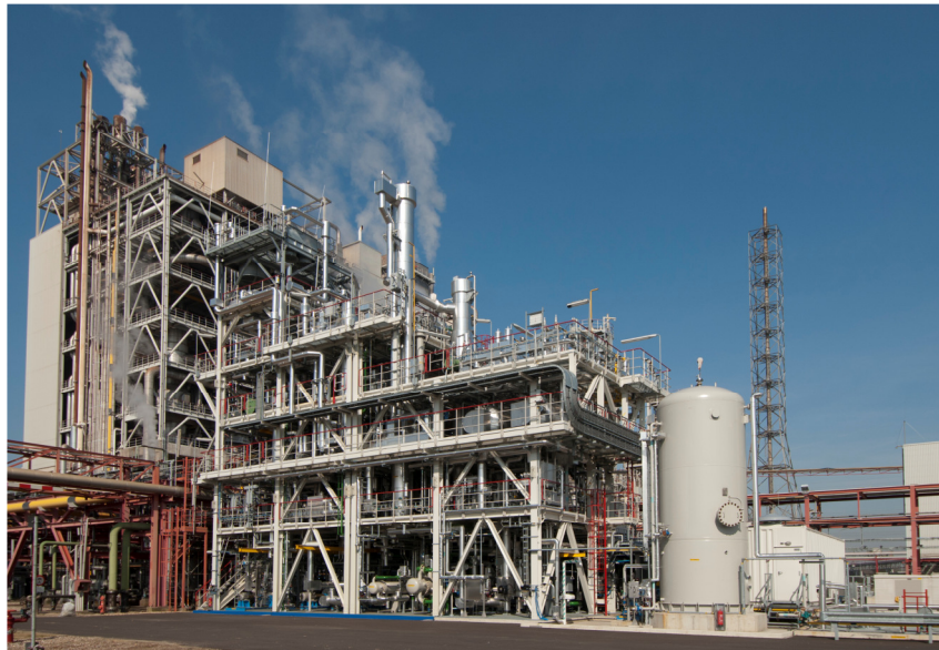
Fig. 2. Picture of the pilot plant at the Buggenum power station
