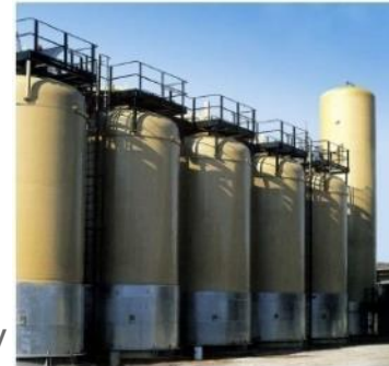
PSA Plant for CO 2 -removal, Vereeniging, South
